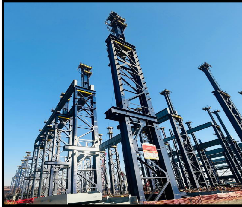
(Heavy Steel fabricated structure built by us at ArcelorMittal Nippon Steel India Ltd., Hazira plant)
